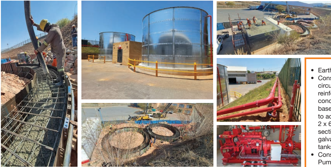
SANLAM PROPERTIES: Calverwall Park Warehouse 1, 2 & 3: Fire Compliance Phase 1 Completed in 2024, Phase 2 completed in 2025
